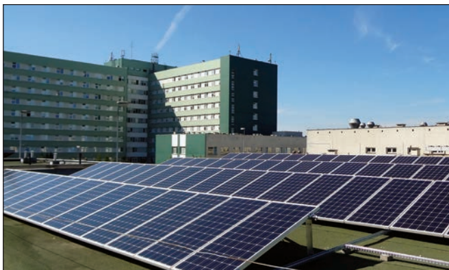
System PV w Radomiu o mocy 21 kWp
